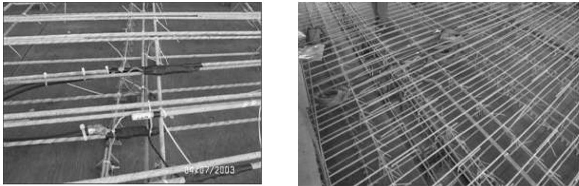
Figure 3.3 Installed civionics instrumentation.
